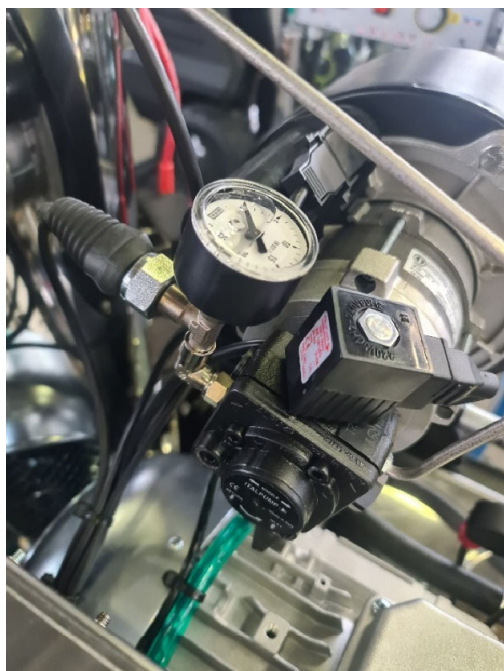
Diesel pump pressure gauge
