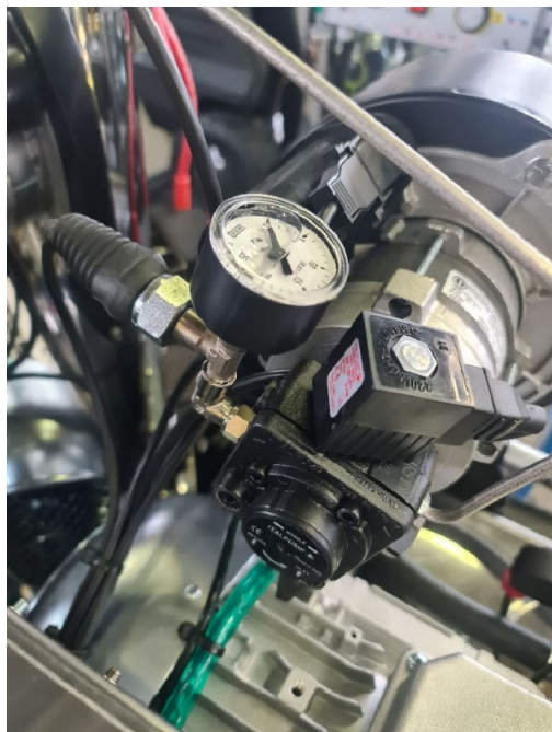
Diesel pump pressure gauge
