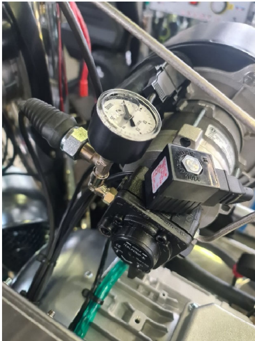
Diesel pump pressure gauge
