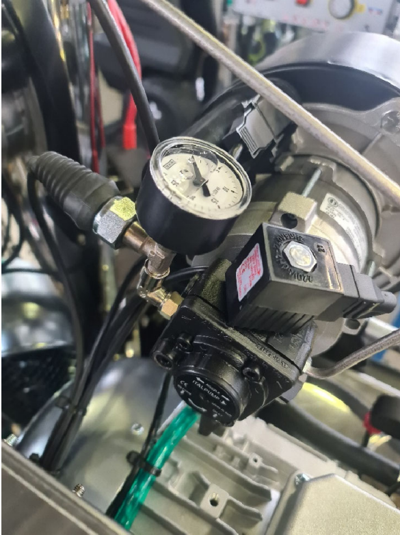
Diesel pump pressure gauge
