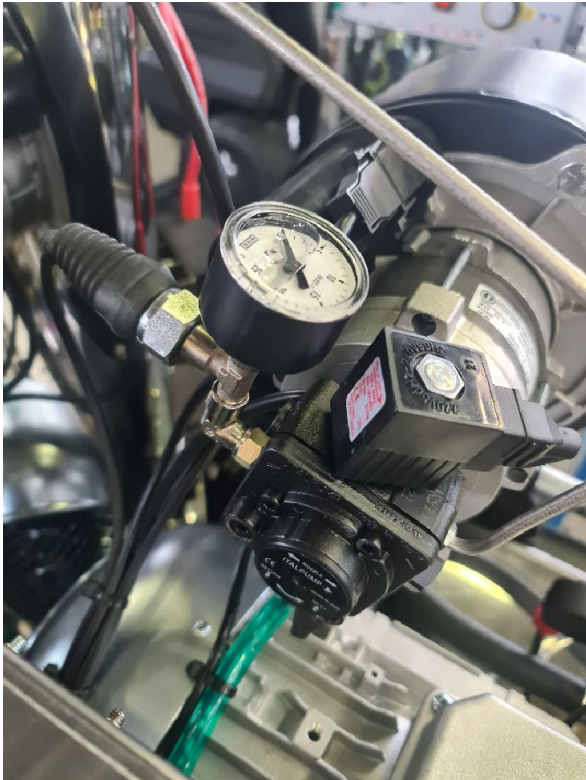
Diesel pump pressure gauge
